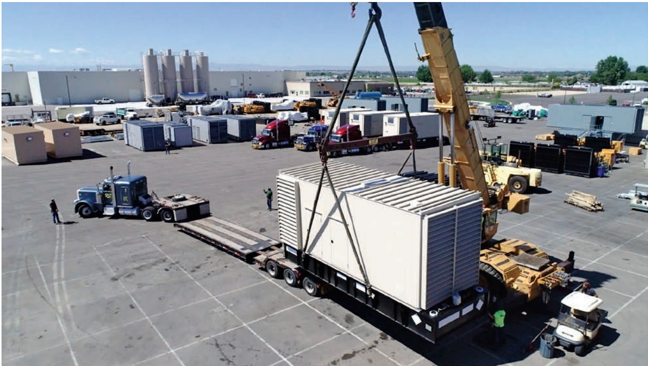
Generator package ready for delivery
