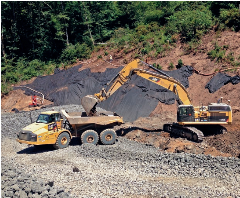
K & E's 374D excavator with 3D GPS machine control near Eddyville, Oregon in 2013
