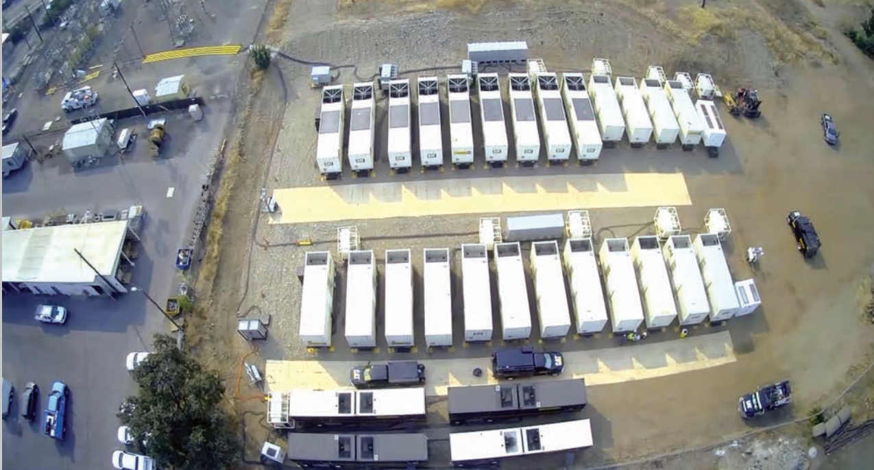
Rental generators onsite in Oroville, California to support Utilities in September 2020
