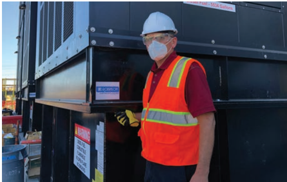
Gene Hamilton at a data center installation in San Jose, California
