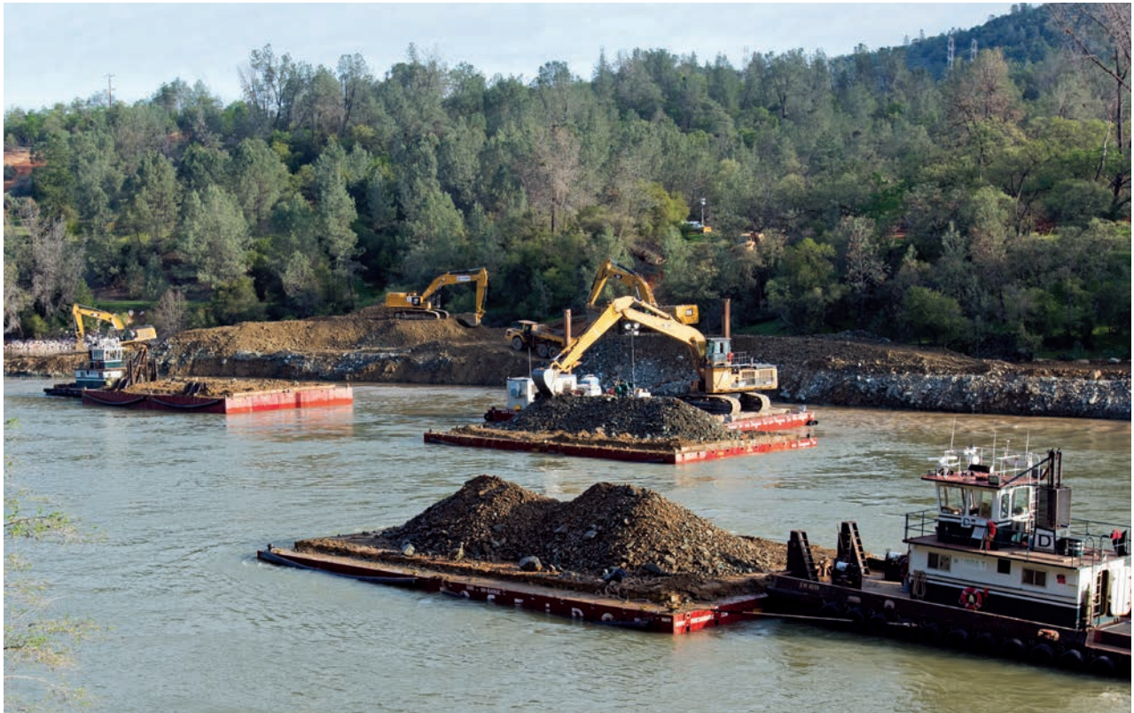
Dredging the Feather River for debris from the spillway break of February 2017
