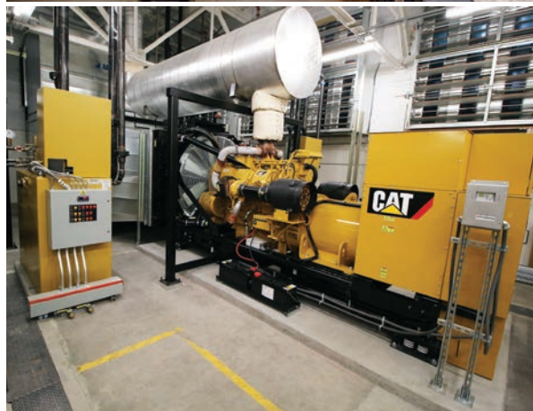
Top to bottom: Cogeneration application at Gresham Wastewater Plant, Oregon in 2015; Standby generator at Good Samaritan Hospital, San Jose, California in 2018
