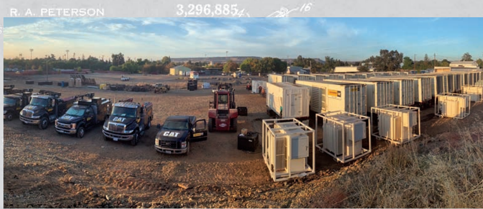
Peterson had 38 MW of prime power in Oroville, CA for the North Complex fire in September 2020
