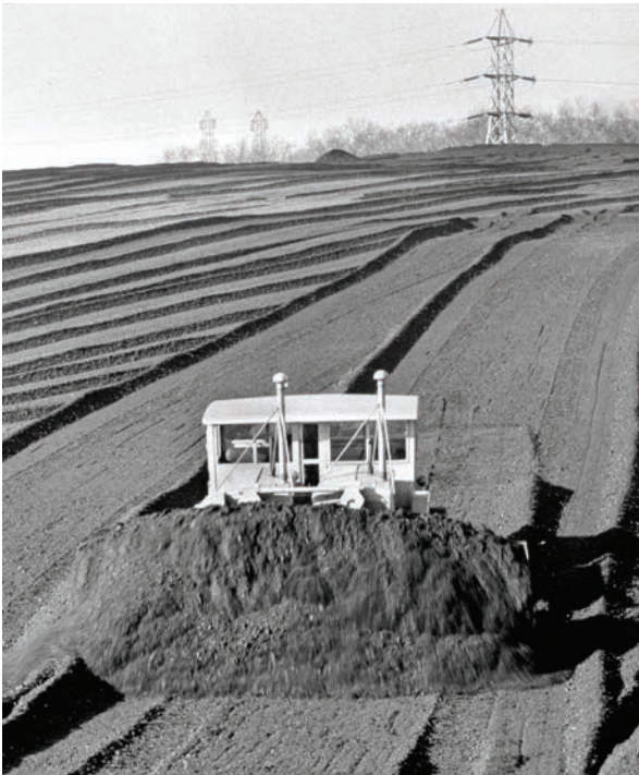
Life Magazine photographer, Andreas Feininger, shot pictures of the Coal Twin at Tanners Creek Power Plant in 1953.
