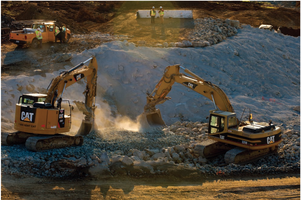
Kiewit orchestrated a massive amount of resources, manpower and logistics to rebuild both Oroville Dam spillways. Teamwork made it happen.
