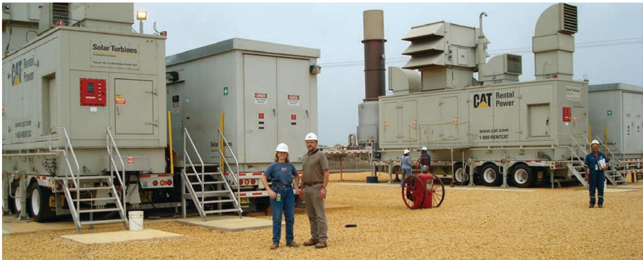
Turbine installation in Cabinda, Angola
