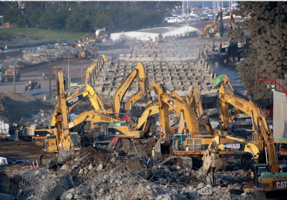
Ferma had 60 excavators on the Doyle Drive contract to beat the clock on the time-sensitive job.
