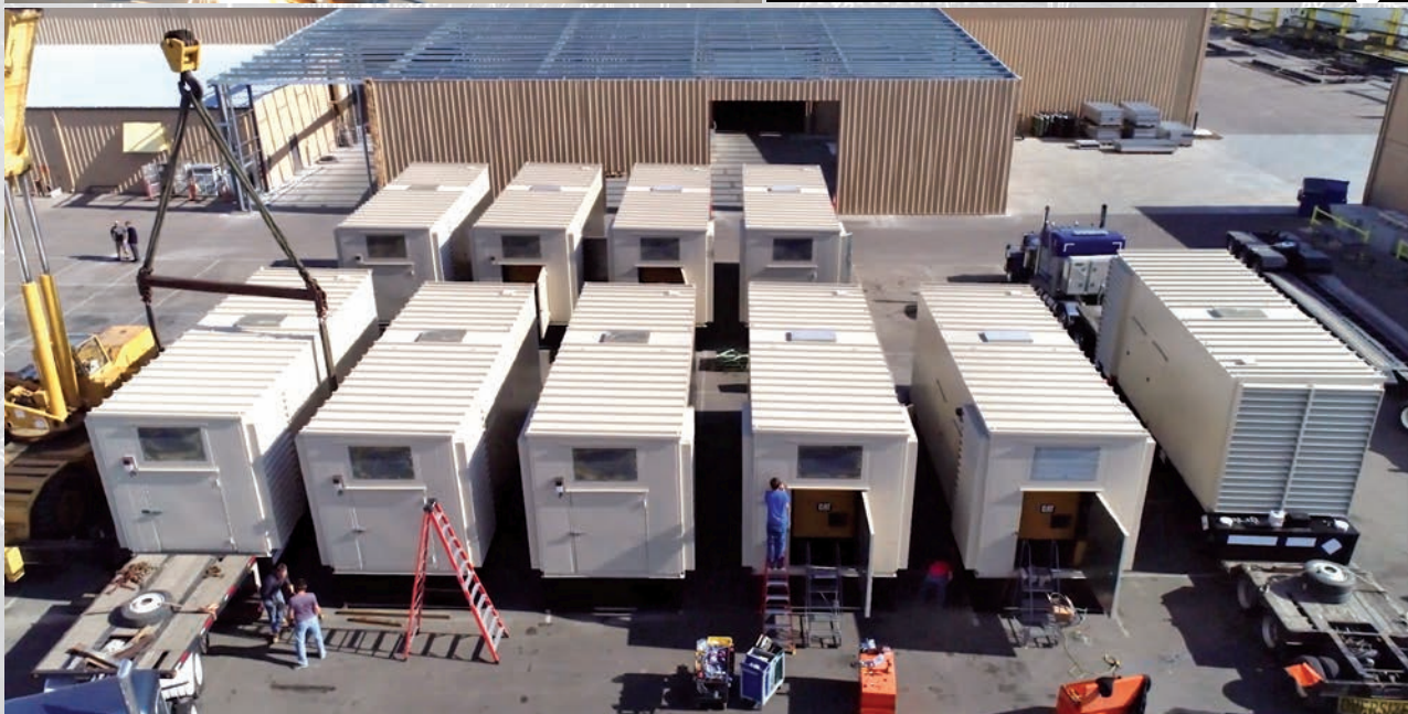
Top to bottom: Welders working on long steel structure; Ten backup generator systems ready to ship from JTS facility in Caldwell, Idaho
