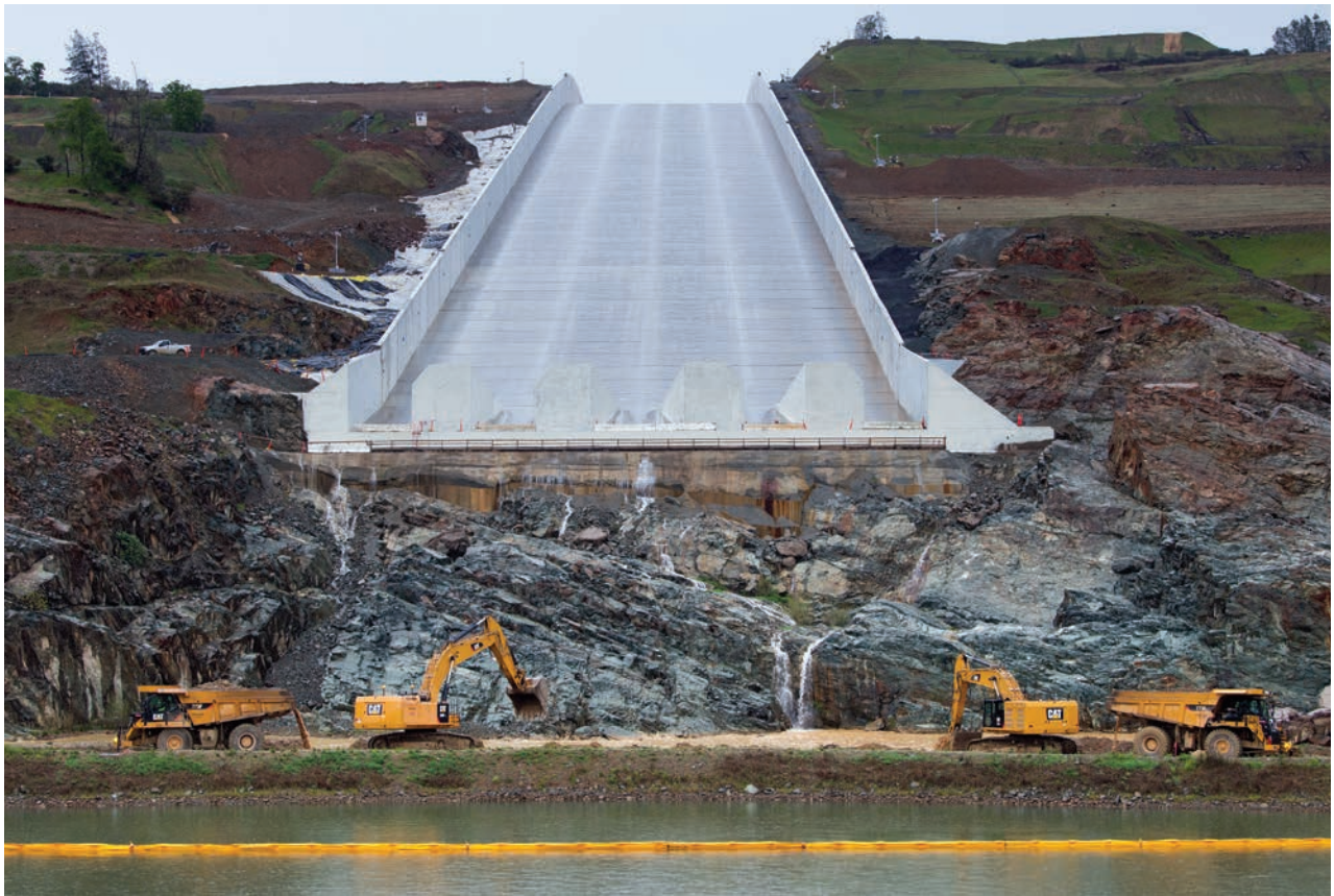
Top to bottom: Oroville Dam's emergency spillway was finished with RCC in a stair-step formation, taken in June 2018; Removal of temporary road just below new main spillway, used during construction, taken in March 2019
