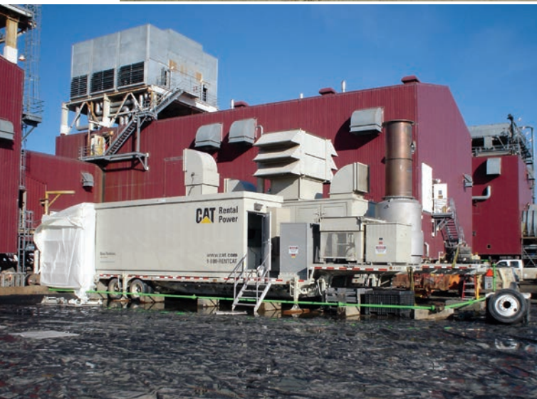
Top to bottom: Jay Pleus at installation in oil fields of Hereford, Colorado; Milne Point installation on the North slope along the Arctic Ocean
