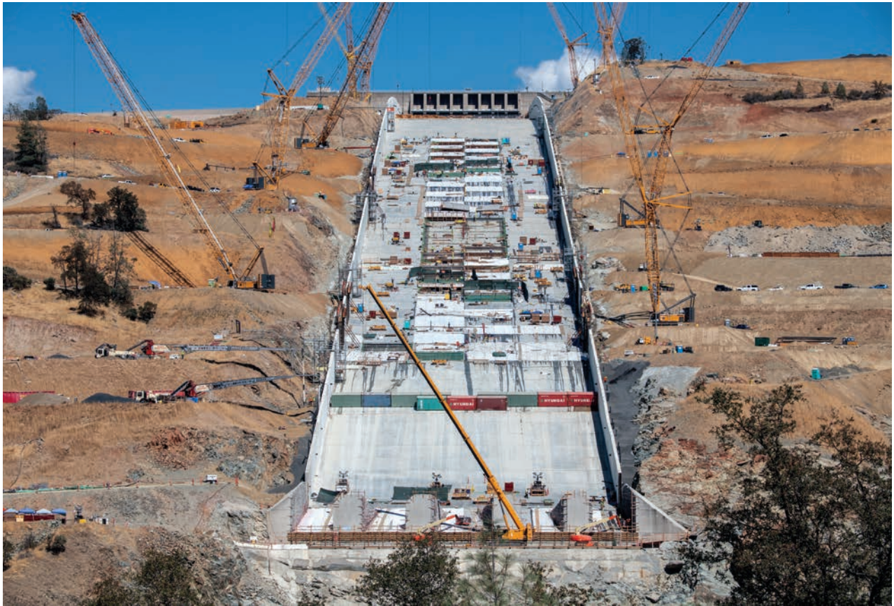
Top to bottom: Main Spillway with Liebherr cranes as transport system in September 2018; Pouring concrete on upper chute of main spillway at night in October 2018; Placing RCC on emergency spillway splash-pad in August 2018
