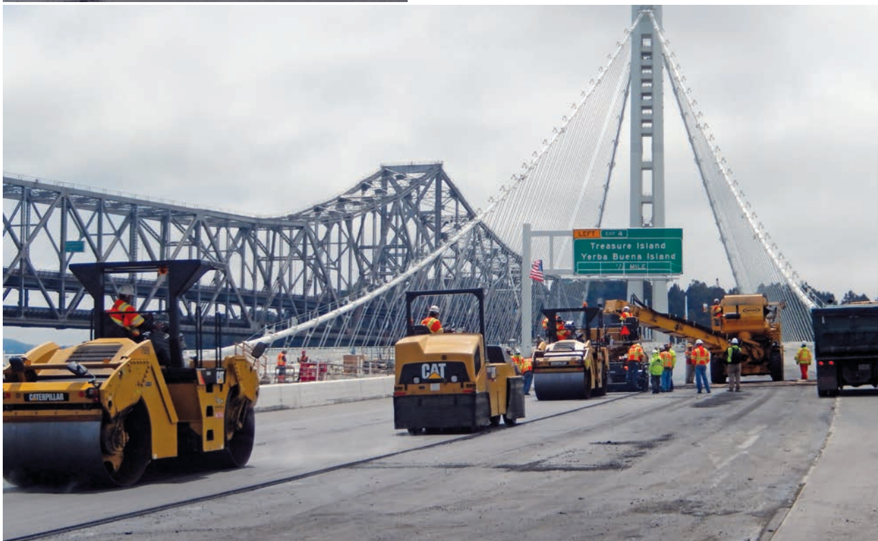
O.C. Jones paved the last section of the SF-Oakland Bay Bridge over Labor Day weekend 2013
