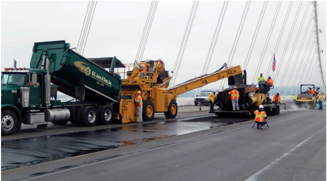
On their Bay Bridge contract in 2013, O.C. Jones ran a Weiler 1250 MTV next to their Cat paver to feed a continuous flow of material into the hopper
