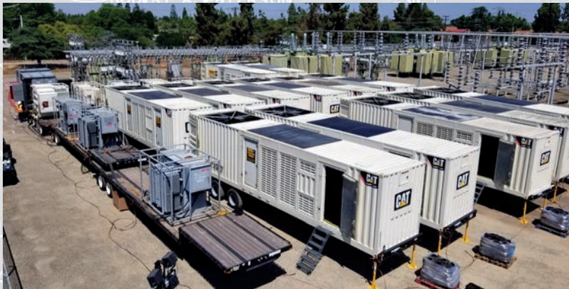
Peterson power modules on rent for utility power
