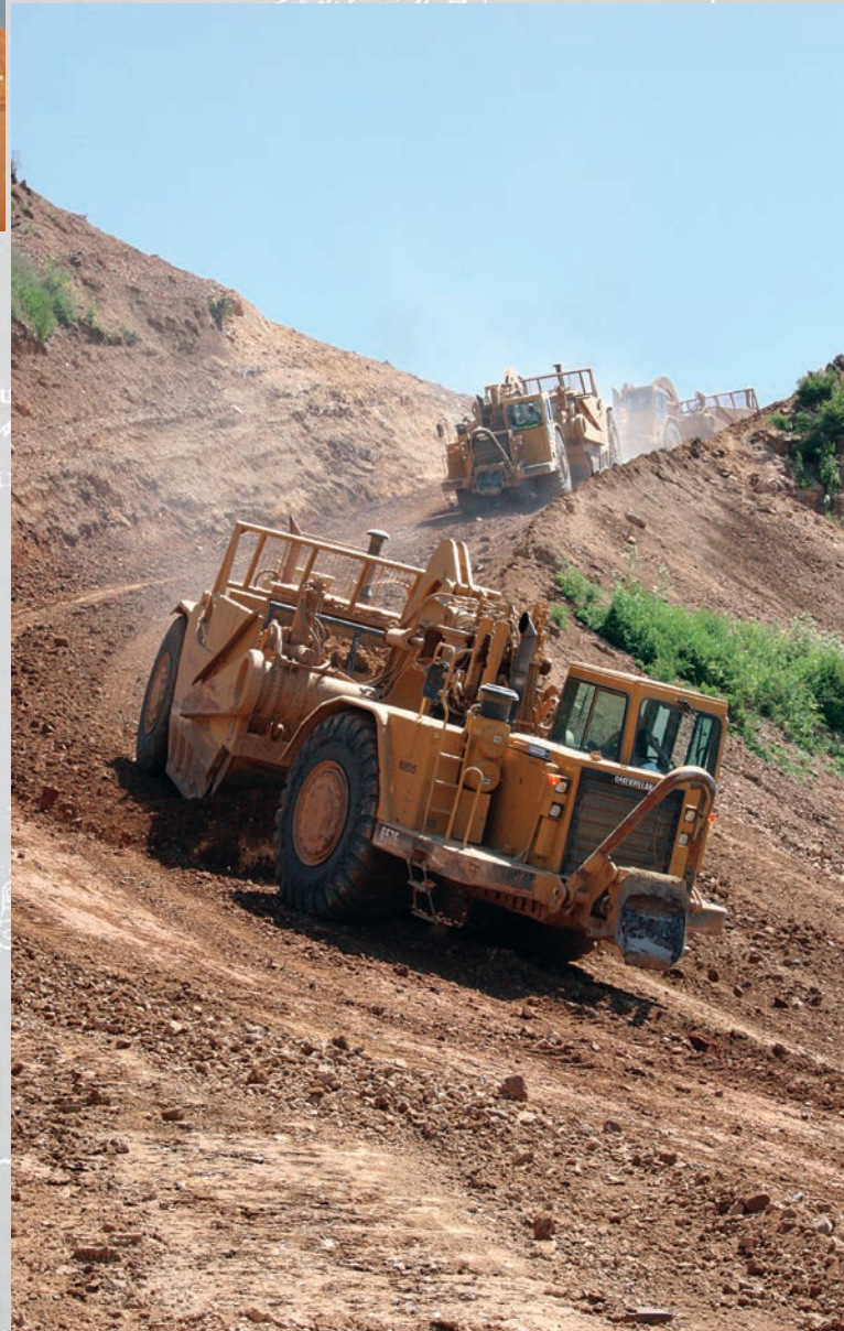
DeSilva scrapers doing site prep at the old Leona Quarry in Oakland, CA circa 2004
