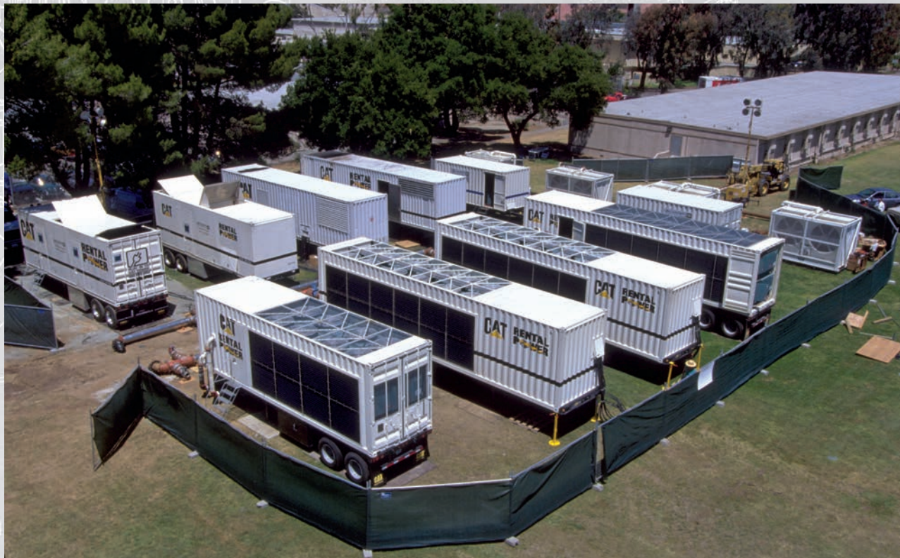
Peterson chillers at Stanford University in Palo Alto, just south of San Francisco.
