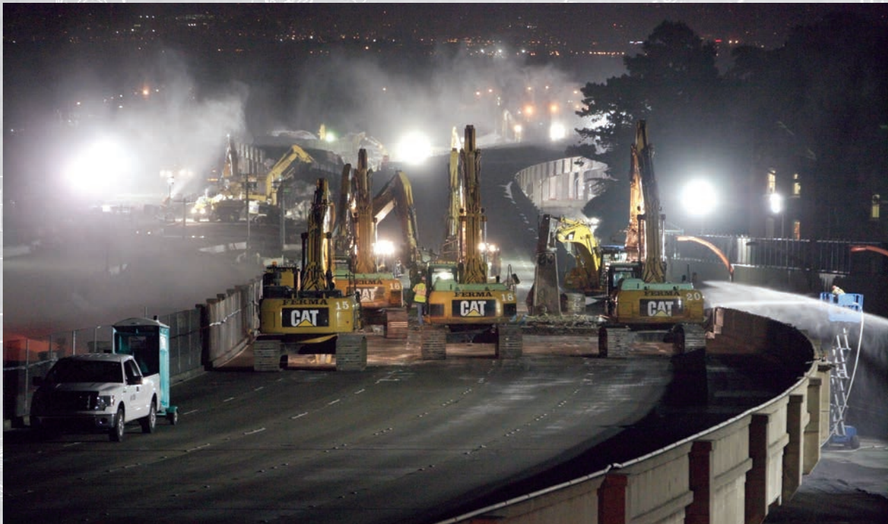
A team of excavators works side by side to demolish Doyle Drive near the San Francisco Presidio in April 2012
