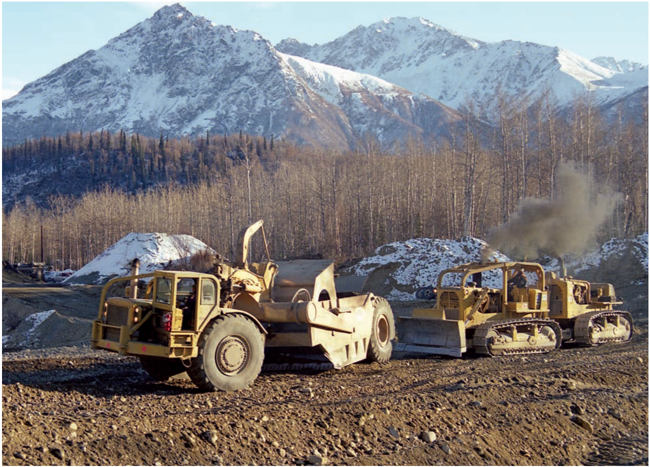
Quad #79 worked on the Glen Hwy in Alaska—from Sutton to King's River—for Wilder Construction in 2000
