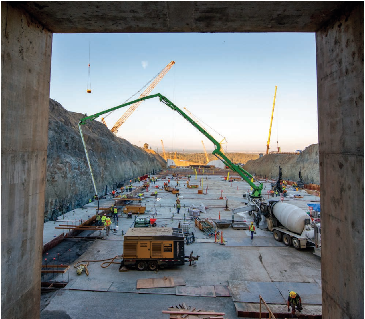
Cat rental generators and air compressors from Peterson helped power Kiewit's jobsite during the spillway project
