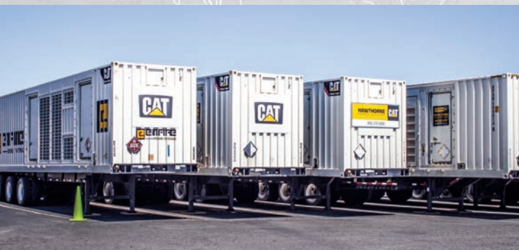
Rental generators from several other Cat dealers waiting in anticipation of the PSPS season in 2020
