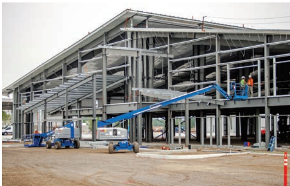
In 2017–18 Peterson built a new facility on 22-acres in Hillsboro, for its Oregon/Washington home base.
