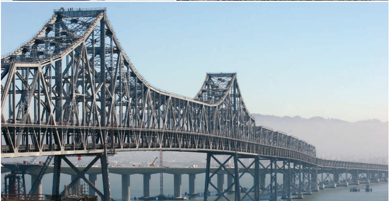
Peterson's support on SF Bay Area bridges through the years. Clockwise from top/left: SF-Oakland Bay Bridge; Benicia-Martinez Bridge; Work on the new & old eastern section of the Bay Bridge.
